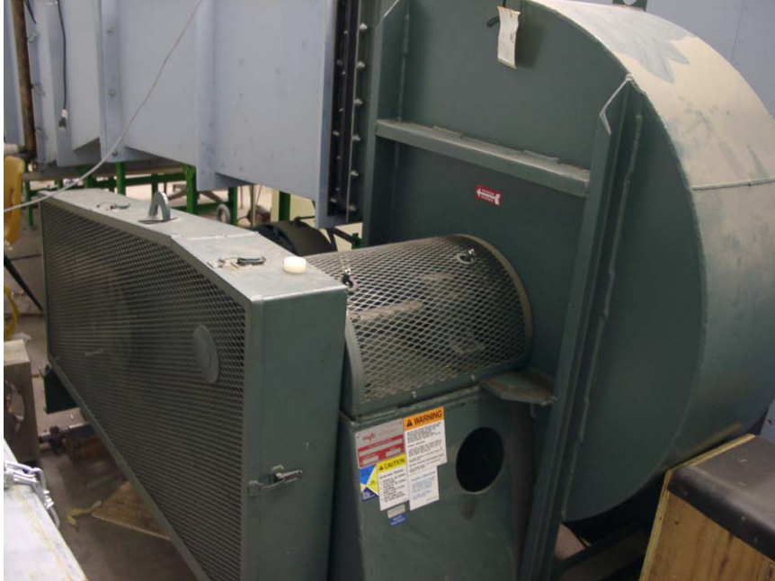
Figure 10. Blower used by UND.
